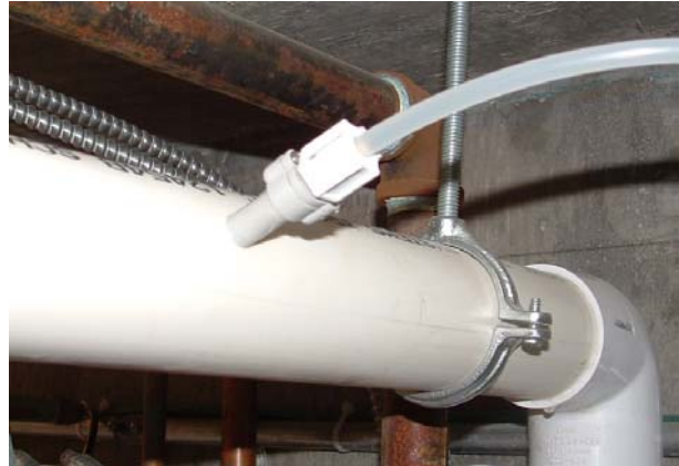
Figure 5a. Discharge tube attached to main feed line
